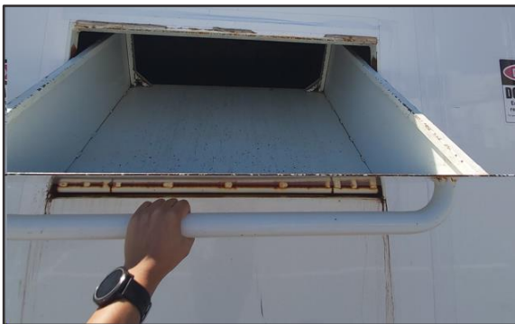
Figure 4: Bucket mechanical chute, rusted over time and difficult to open.
