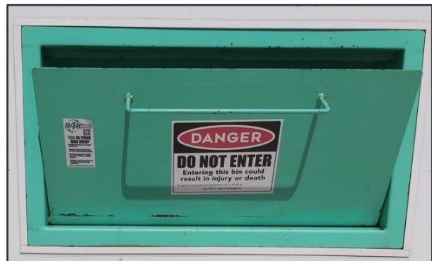
Figure 5: Bucket mechanical chute, jammed open due to stuck bag, resulting in limited capacity.
